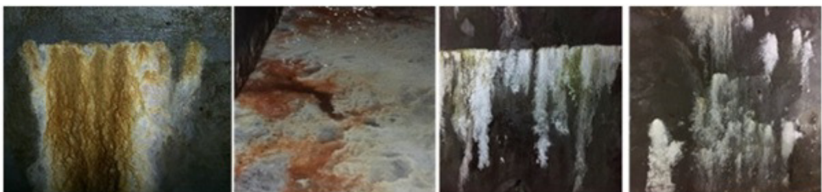
Plate 1: Photographs of Foundation galleries of Baglihar HEP showing the leaching of lime
