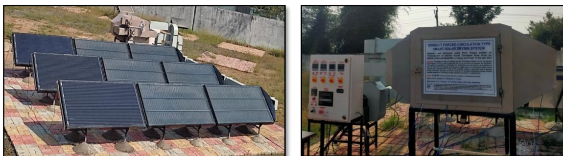
Fig.2: PV-thermal and packed bed collectors with drying chamber, control panel, ducting and blower
